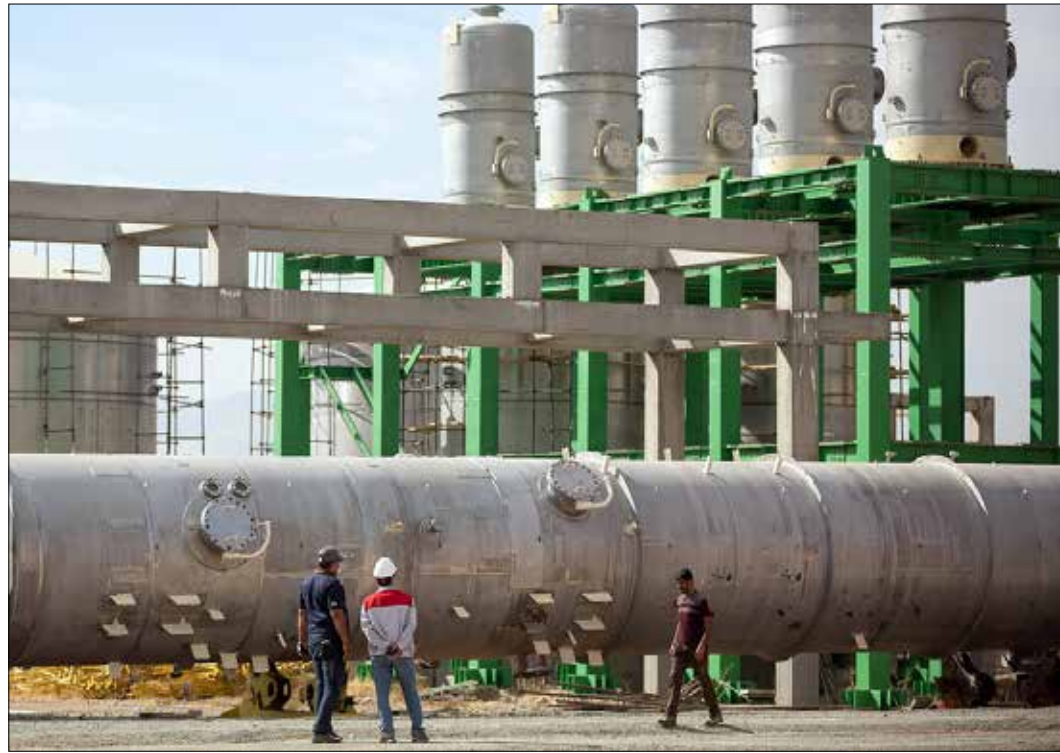
Persian Gulf Bid Boland Gas Refining Company in southwestern Iranian province of Khuzestan
